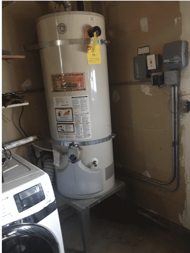
Today: 50-gallon gas tank WH in garage
