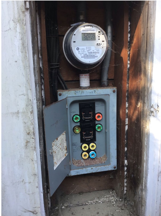
Today: 100-amp fuse box
